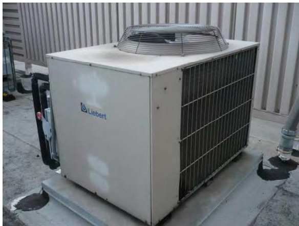
Rooftop Air Conditioner
