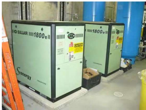
Support Equipment - Compressed Air System
