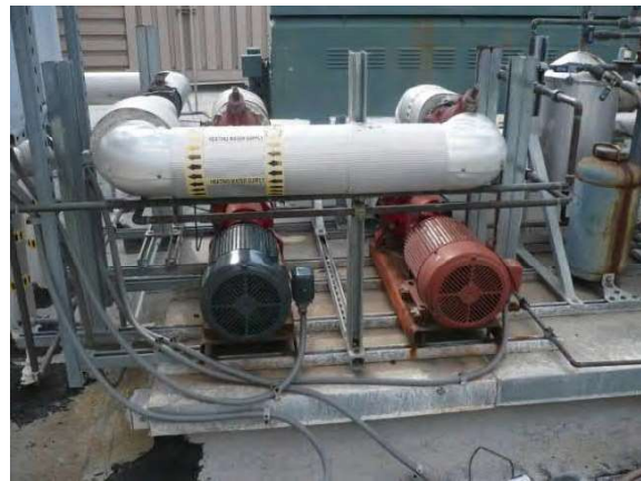
Hot Water Recirculation Pumps
