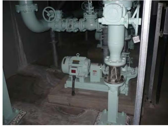
Service Water Pump
