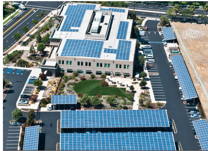
Solar panels at San Diego Headquarters Building
