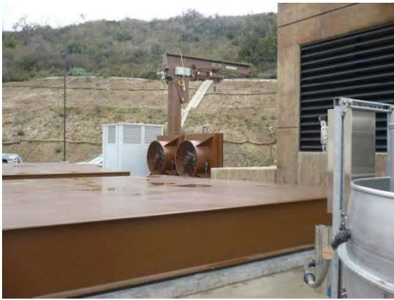
Top Hatch of Pump/Generator Station
