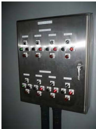
Service/Cooling Water Panel
