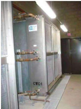
Cooling Water System
