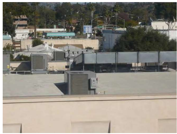
Rooftop Mechanical Equipment
