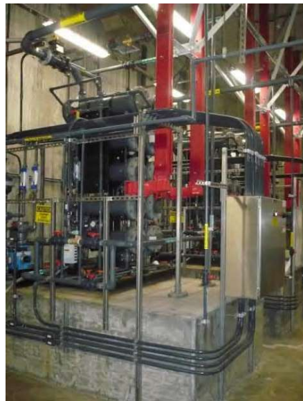
Sodium Hypochlorite Generation System
