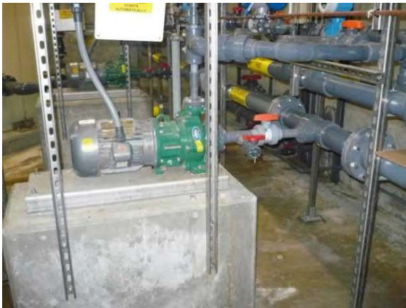
Chemical Water Mixing Pumps
