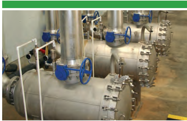
Sweetwater Authority's Richard A. Reynolds Groundwater Desalination Facility
