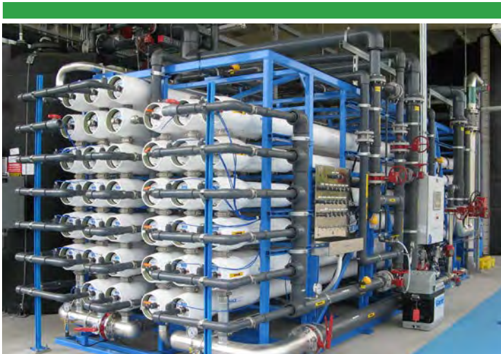
Reverse osmosis technology at the City of San Diego’s North City Water Reclamation Plant
