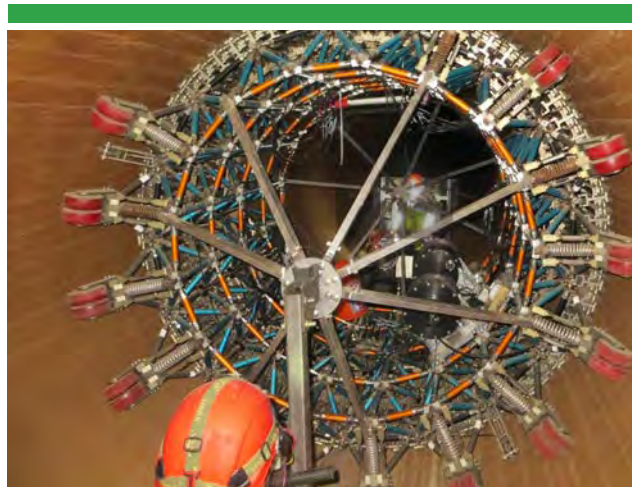
Crews inspect the integrity of the water distribution system using the most current technologies.
