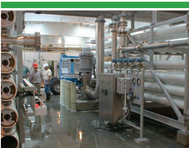
The City of Oceanside's Mission Basin Brackish Groundwater Desalting Demonstration Project received $3.484 million in funding.
