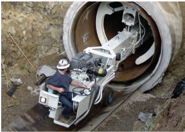
Asset management efforts include pipeline relining to extend the life of the aging infrastructure.
