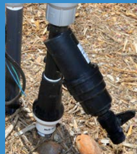
4 pressure regulator and filter for drip irrigation
