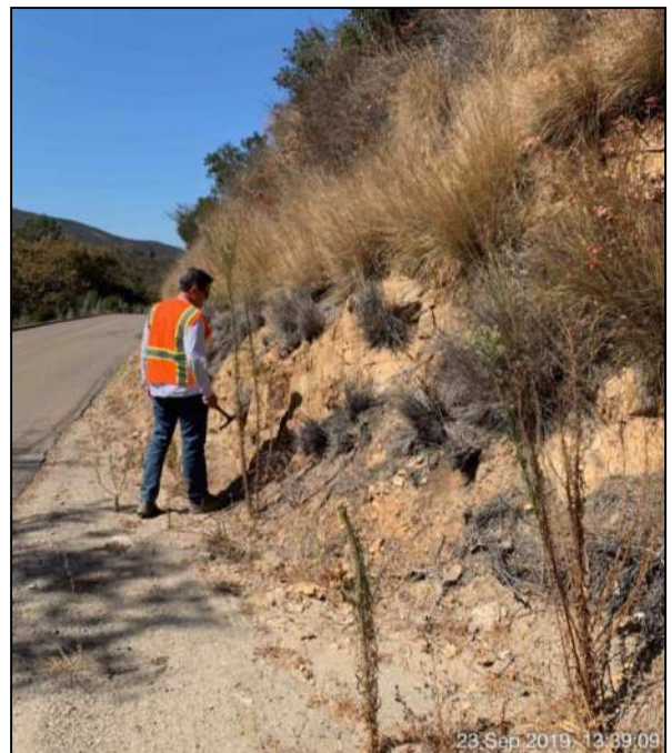
PHOTO 236: Cut of highly weathered granite along east side of Twin Oaks Valley Road near TOVWTP.
