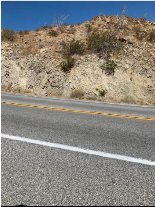
PHOTO 73: Sheared rock likely due to nearby faulting.
