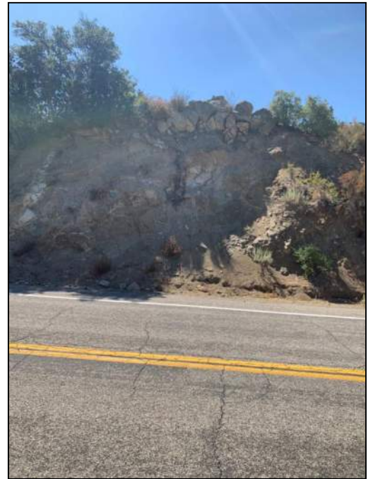
PHOTO 152: Cut on south side of S22 west of Ranchita.
