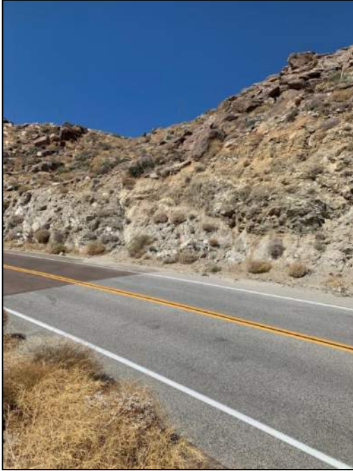
PHOTO 105: Highly weathered and fractured granitic rock.
