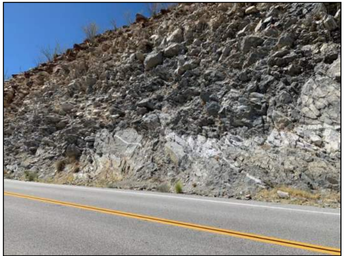
PHOTO 84: Highly fractured granitic rock in road cut.
