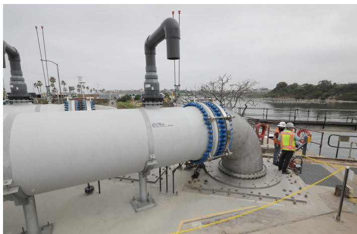
Claude “Bud” Lewis Carlsbad Desalination Plant intake piping, 2020
