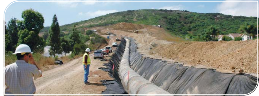
39 Miles of Buried Pipelines
