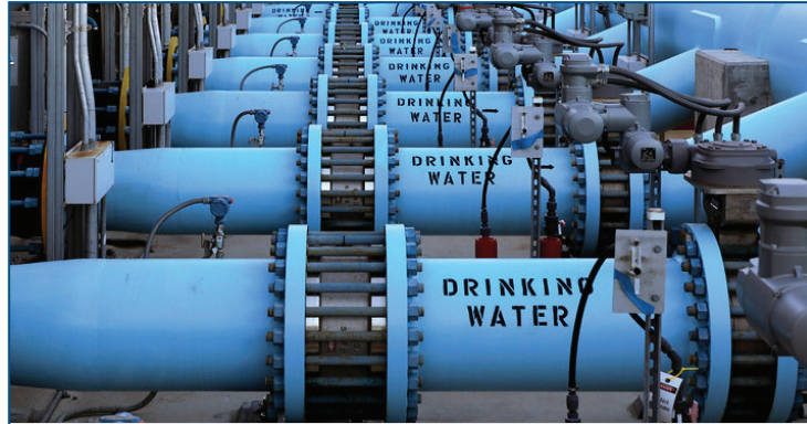
Seawater desalination at the Claude "Bud" Lewis Carlsbad Desalination Plant can provide up to 56,000 AFY of a highly reliable, drought-proof supply for the region.
