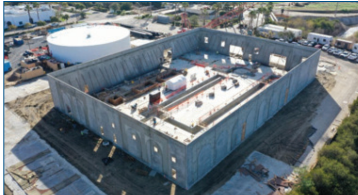
Pure Water Oceanside, which is currently under construction, will augment groundwater supply in the Mission Basin. Photo credit: City of Oceanside
