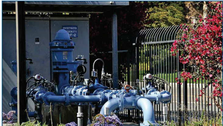
High quality groundwater extraction wells contribute to the Sweetwater Authority's potable water supply.
