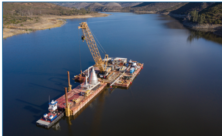
The Hodges Reservoir Hypolimnetic Oxygenation System, or Speece cone, provides a very efficient method for increasing oxygen levels in Lake Hodges Reservoir, supporting improved water quality.
