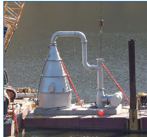
Example IRWM Project: The Hodges Reservoir Hypolimnetic Oxygenation System, or Speece Cone, was installed to oxygenate water at the bottom of Hodges Reservoir to support improved water quality in the reservoir. This will allow for reduced treatment cost of water from the reservoir, as well as expand the uses of water stored in Hodges Reservoir.
