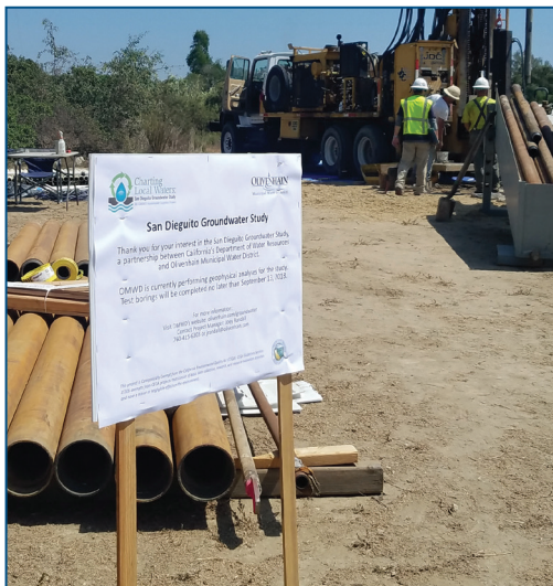
Drilling a pilot well was the first step of the San Dieguito River Basin Brackish Groundwater Recovery Project, a conceptual potable reuse project. Photo credit: Olivenhain Municipal Water District
