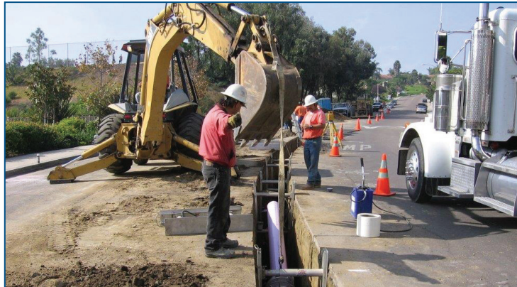
The IRWM Program has supported recycled water expansion through the North San Diego Regional Recycled Water Program, an ongoing partnership of water and wastewater agencies.
