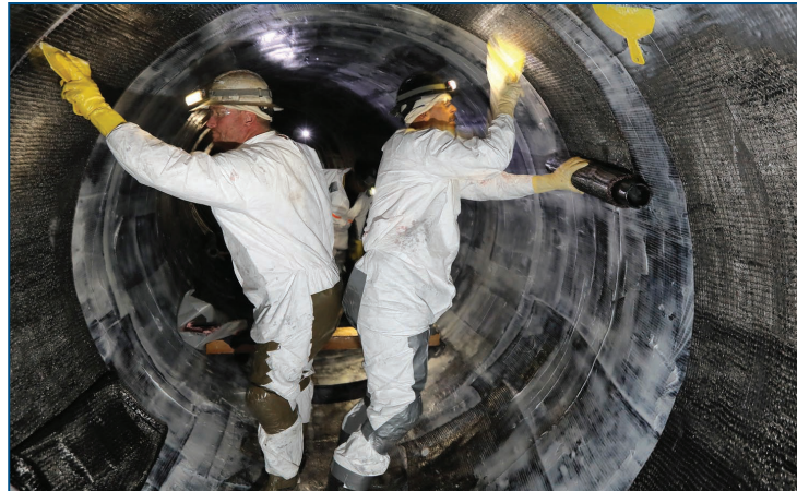
Asset management efforts include pipeline relining to extend the life of infrastructure.
